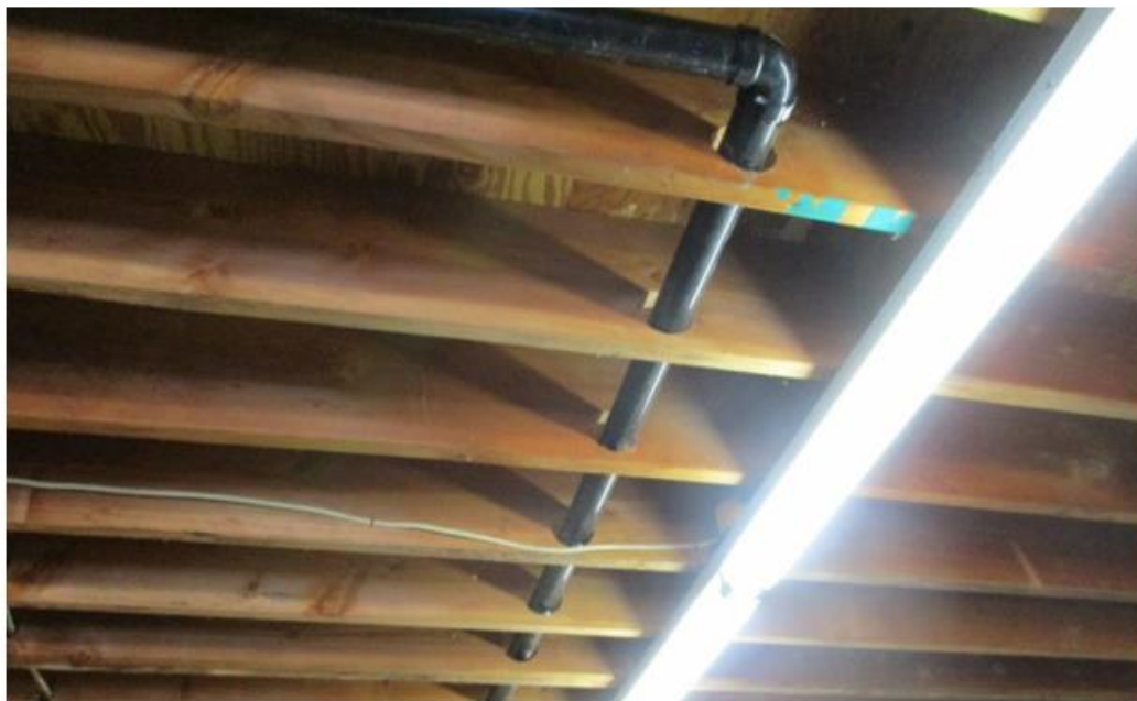
Figure 2.15. Holes Drilled in Joists
