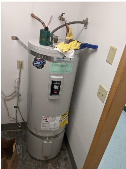
Figure 4.8. Building A Domestic Water Heater
