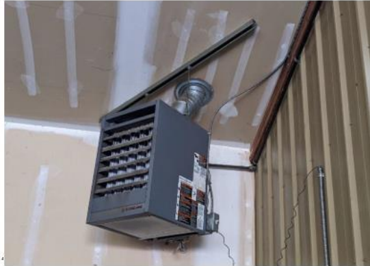
Figure 4.17. Building E Unit Heater
