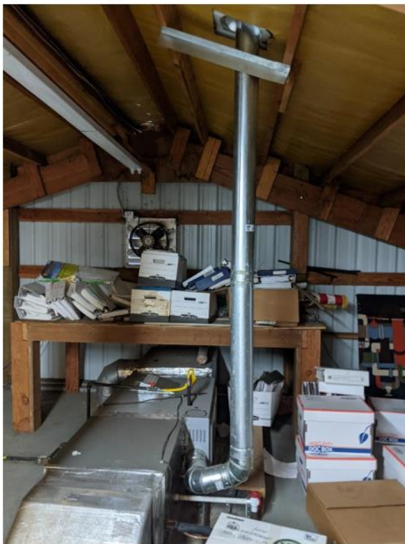
Figure 4.9. Building C Furnace
