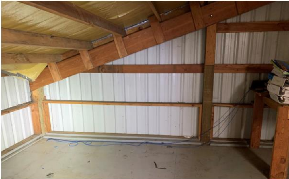
Figure 3.7. Communication Cables in Loft Space
