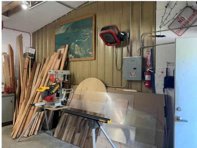
Figure 3.12. Scrap Materials Stored in Front of Panel
