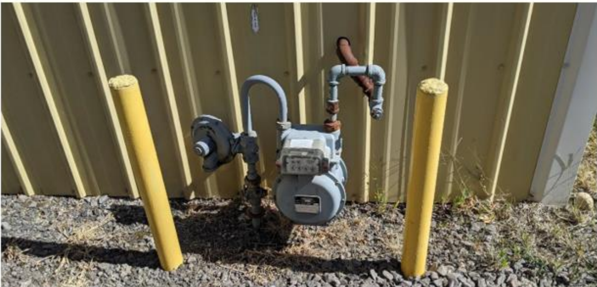
Figure 4.16. Building D Natural Gas Meter
