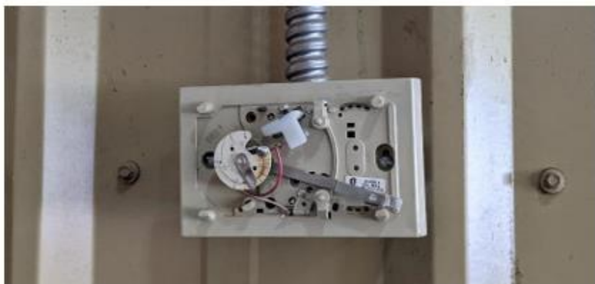
Figure 4.18. Building E Thermostat
