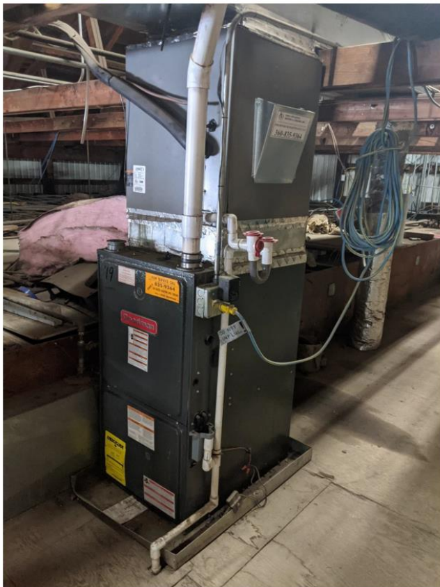
Figure 4.2. Building A Admin A/C
