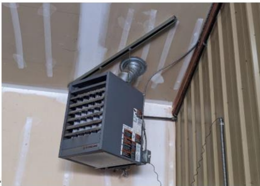
Figure 4.17. Building E Unit Heater
