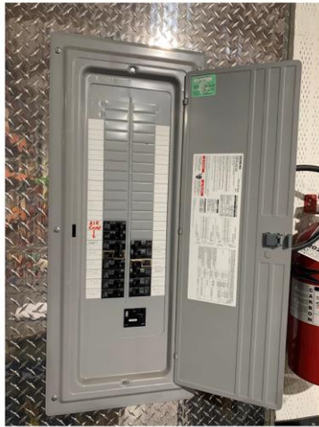
Figure 3.13. Building G Panel
