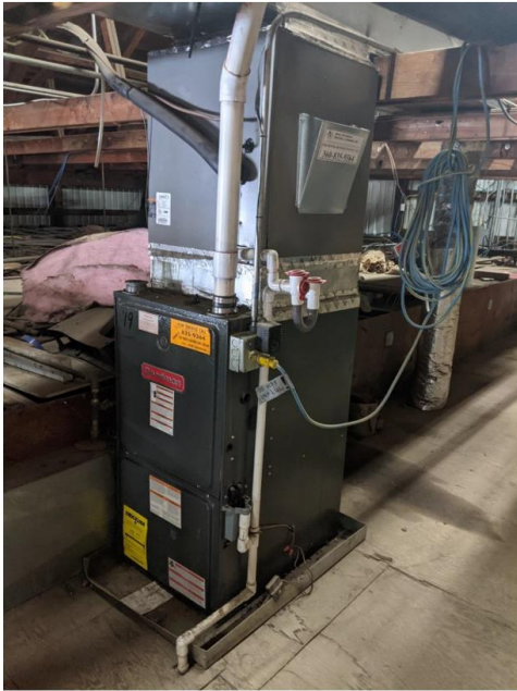
Figure 4.1. Building A Admin Furnace
