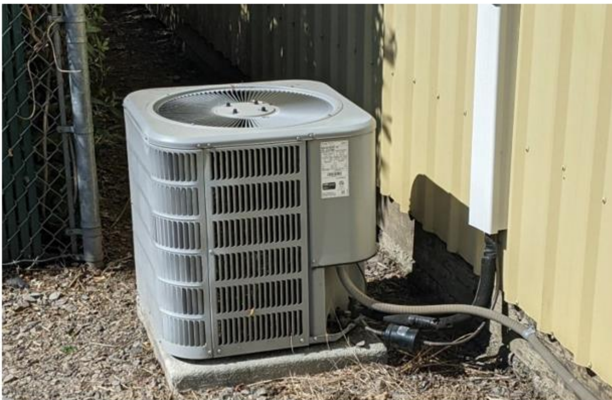
Figure 4.10. Building C A/C
