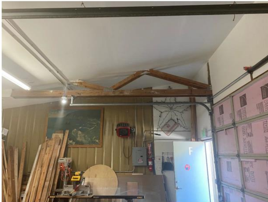
Figure 2.20. Roof Structure Hidden with Drywall
