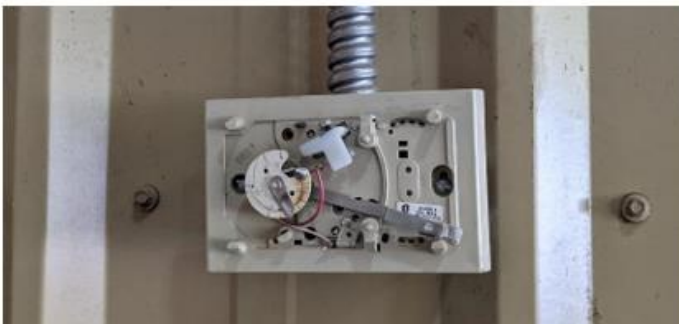
Figure 4.18. Building E Thermostat
