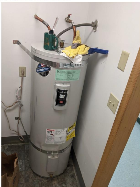
Figure 4.8. Building A Domestic Water Heater
