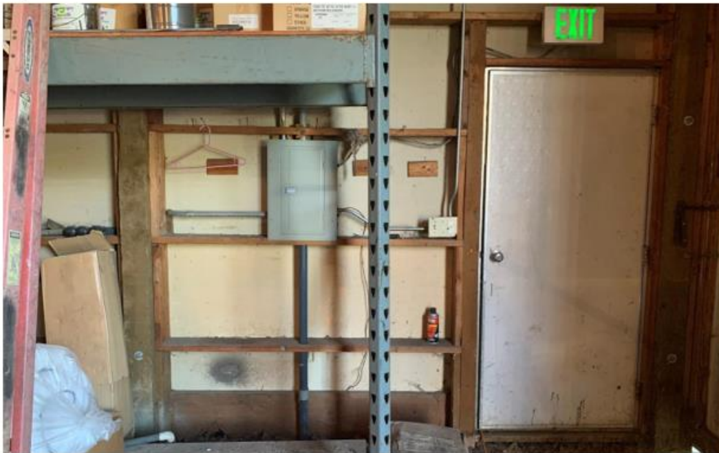
Figure 3.10. Metal Shelf in Front of Panel
