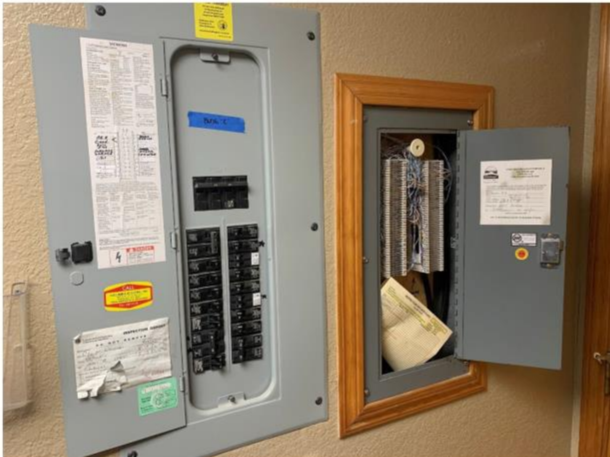
Figure 3.5. Building C Panelboard
