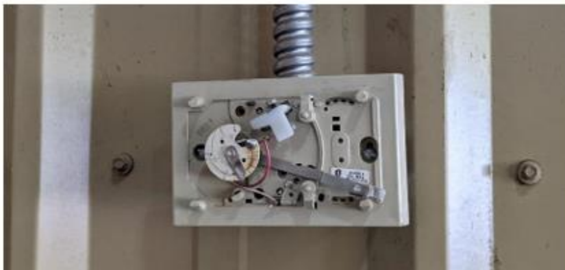
Figure 4.18. Building E Thermostat
