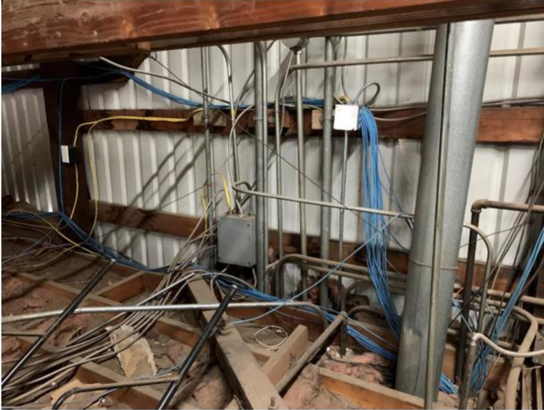
Figure 3.4. Communication Cables in Attic
