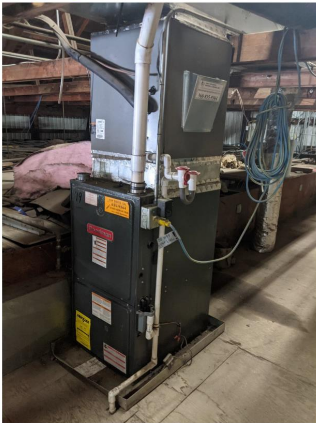
Figure 4.2. Building A Admin A/C
