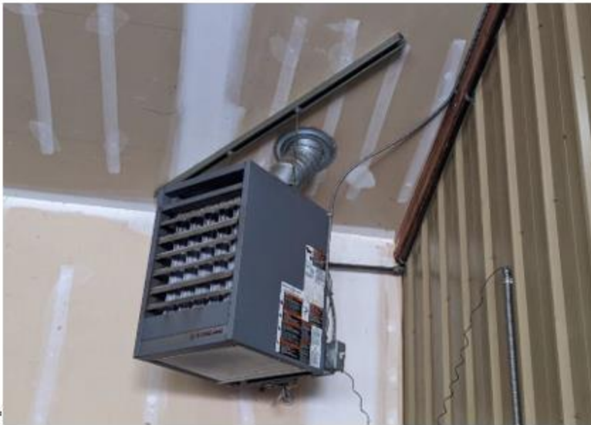
Figure 4.17. Building E Unit Heater
