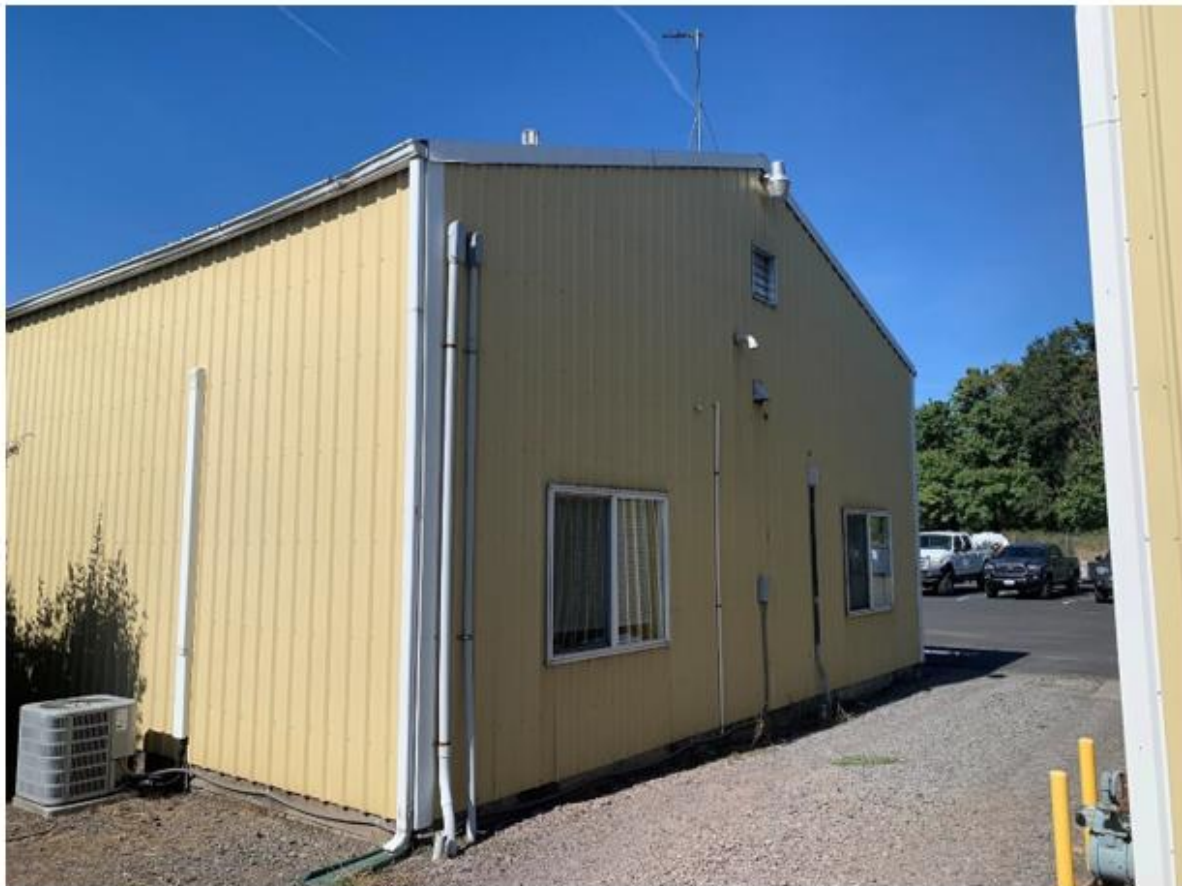
Figure 3.8. HVAC Unit and Disconnect Switch
