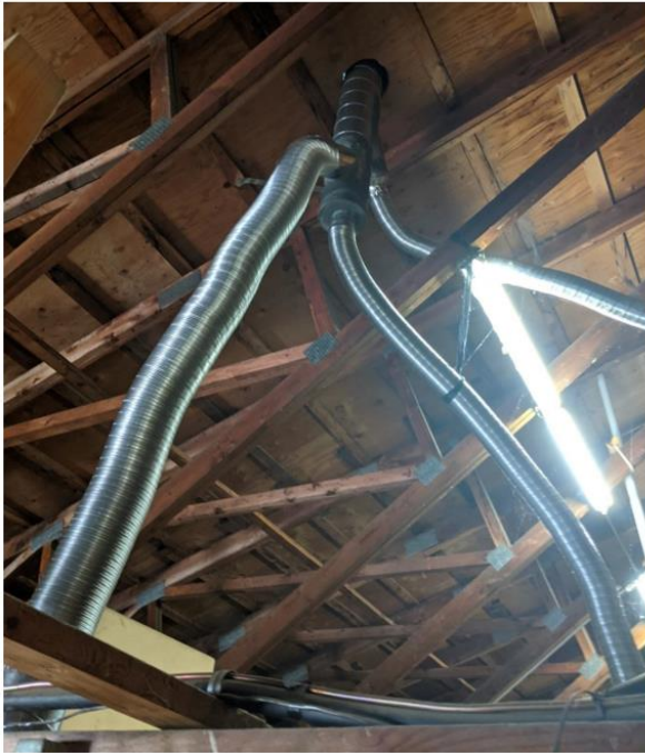
Figure 4.7. Building A Exhaust Connections
