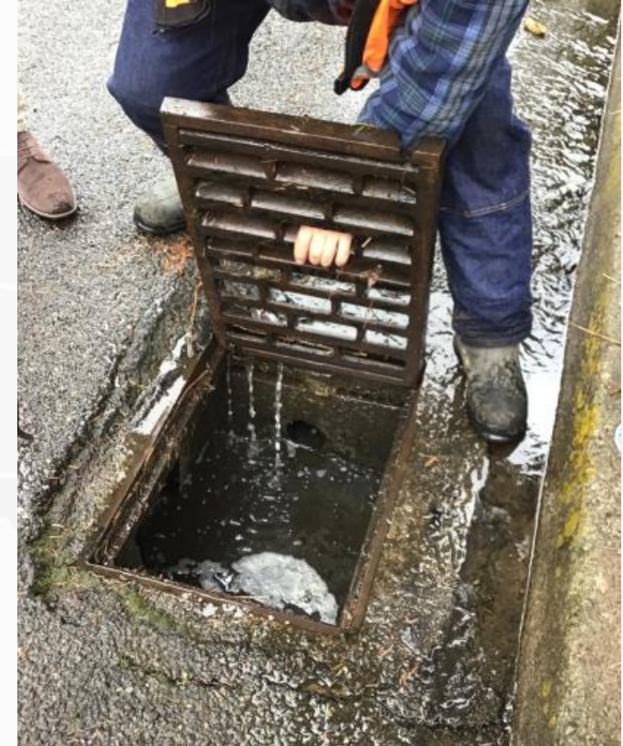
Non-standard structures, low inlet capacity
