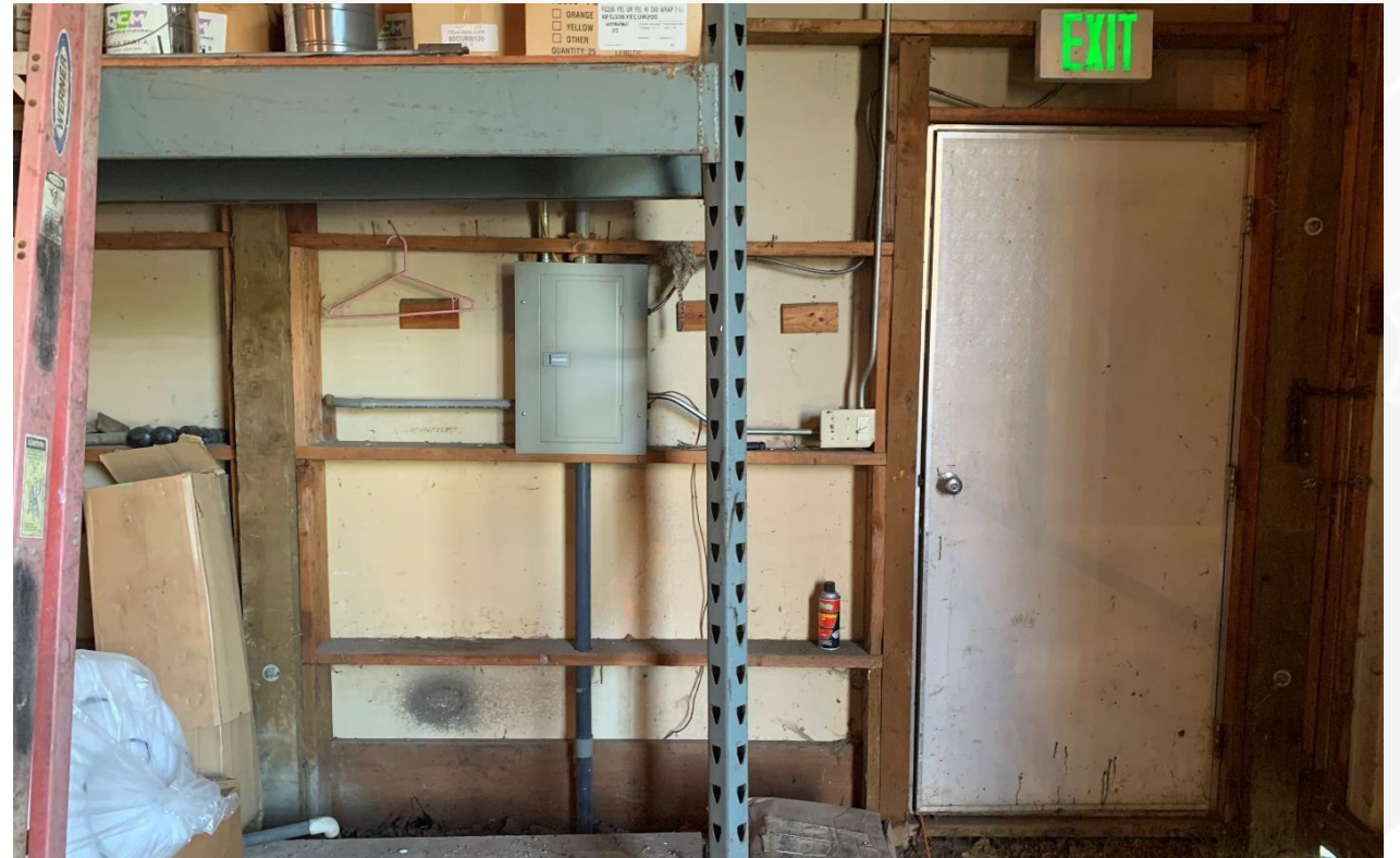
Figure 3.10. Metal Shelf in Front of Panel
