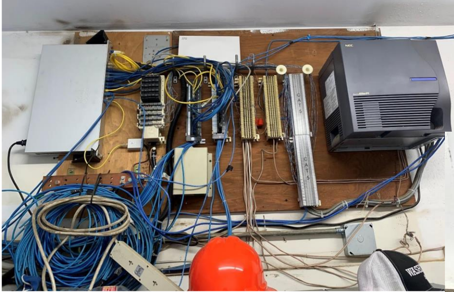
Figure 3.3. Exposed Communication Equipment
