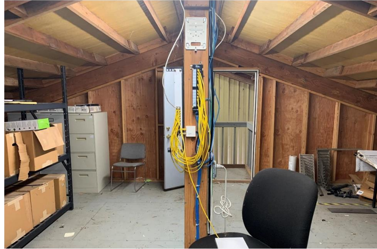
Figure 3.6. Networking hardware in Loft
