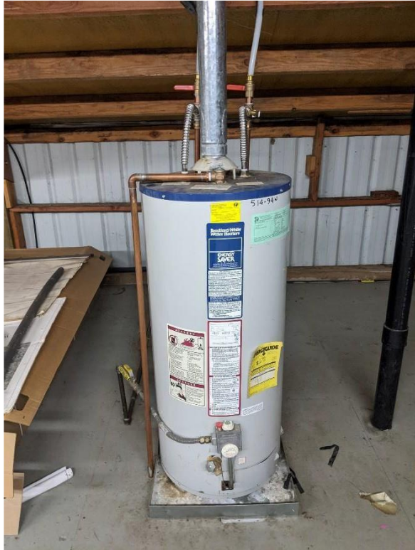
Figure 4.14. Building C Domestic Water Heater
