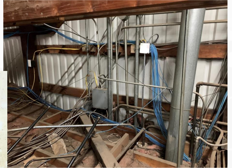
Figure 3.4. Communication Cables in Attic
