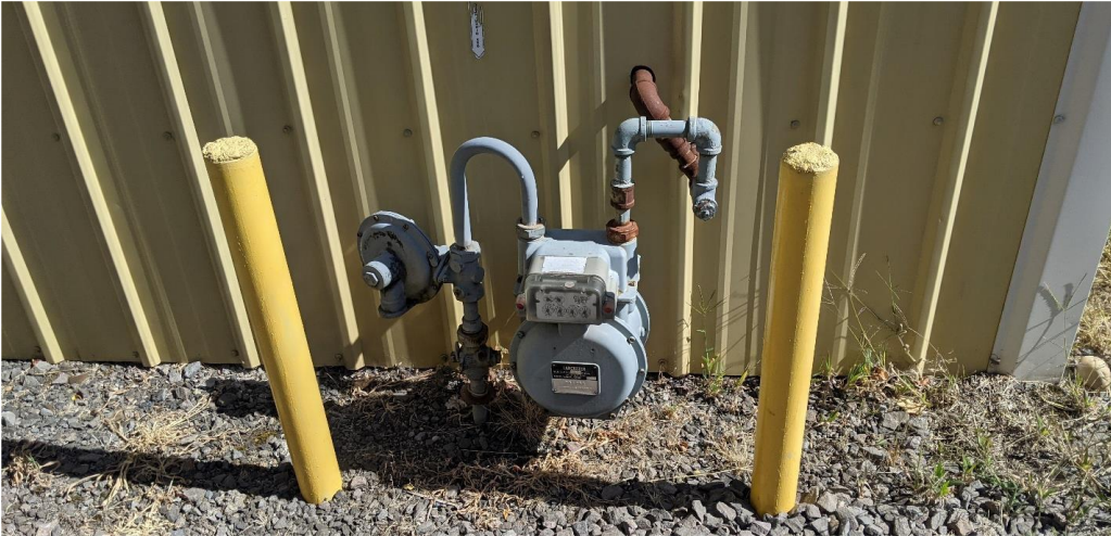
Figure 4.16. Building D Natural Gas Meter
