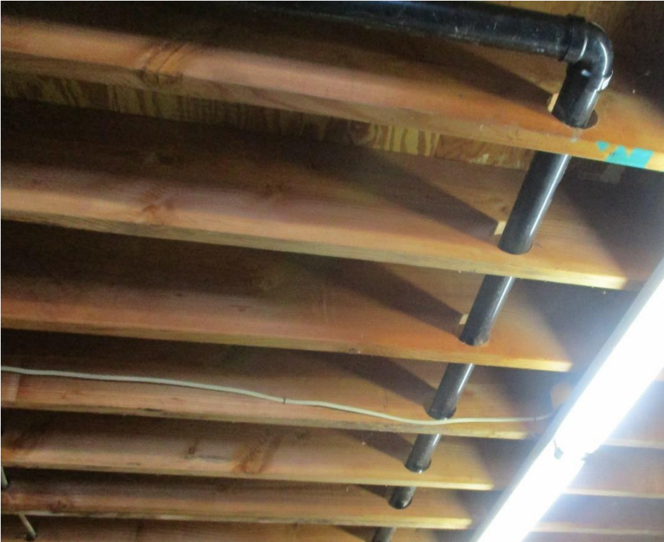
Figure 2.15. Holes Drilled in Joists
