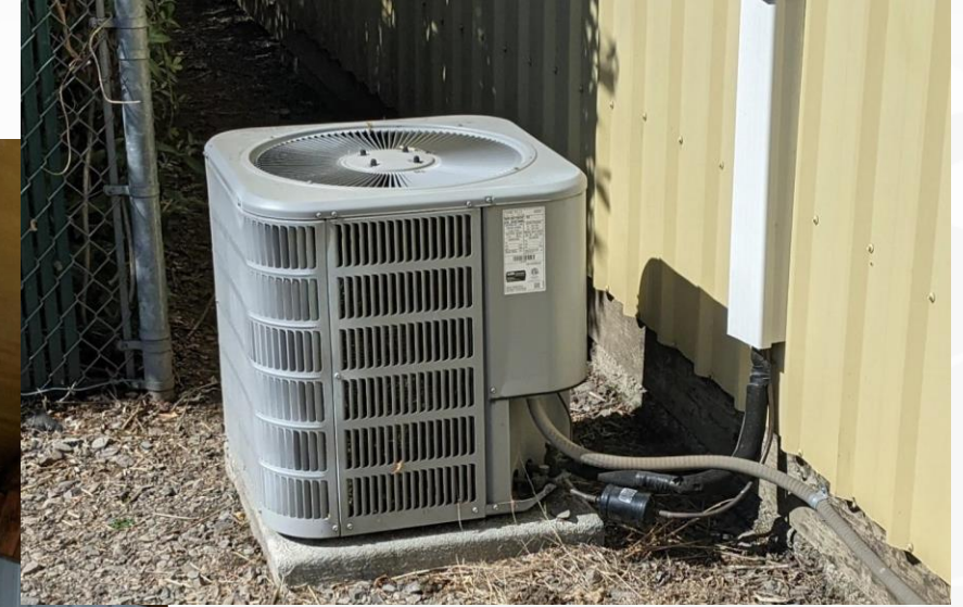
Figure 4.10. Building C A/C
